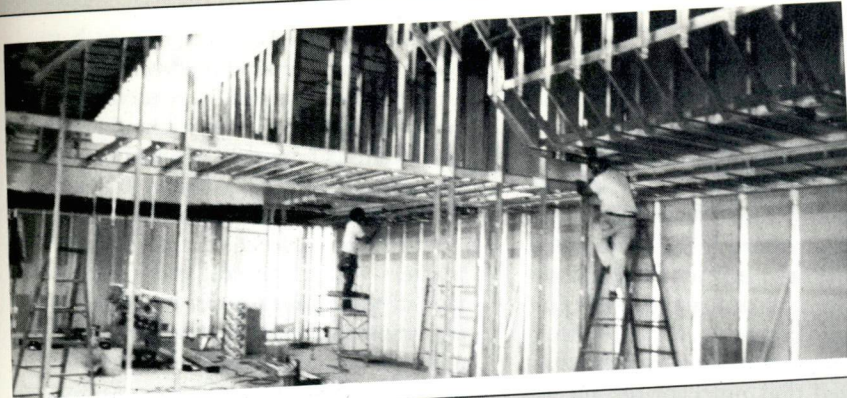
Board room's skeleton —This is the former atrium from the same angle as the photo at left—only now glass walls have been replaced with the structural skeleton of a new Board room. The rectangular slice of light in the ceiling is the skylight opening.
